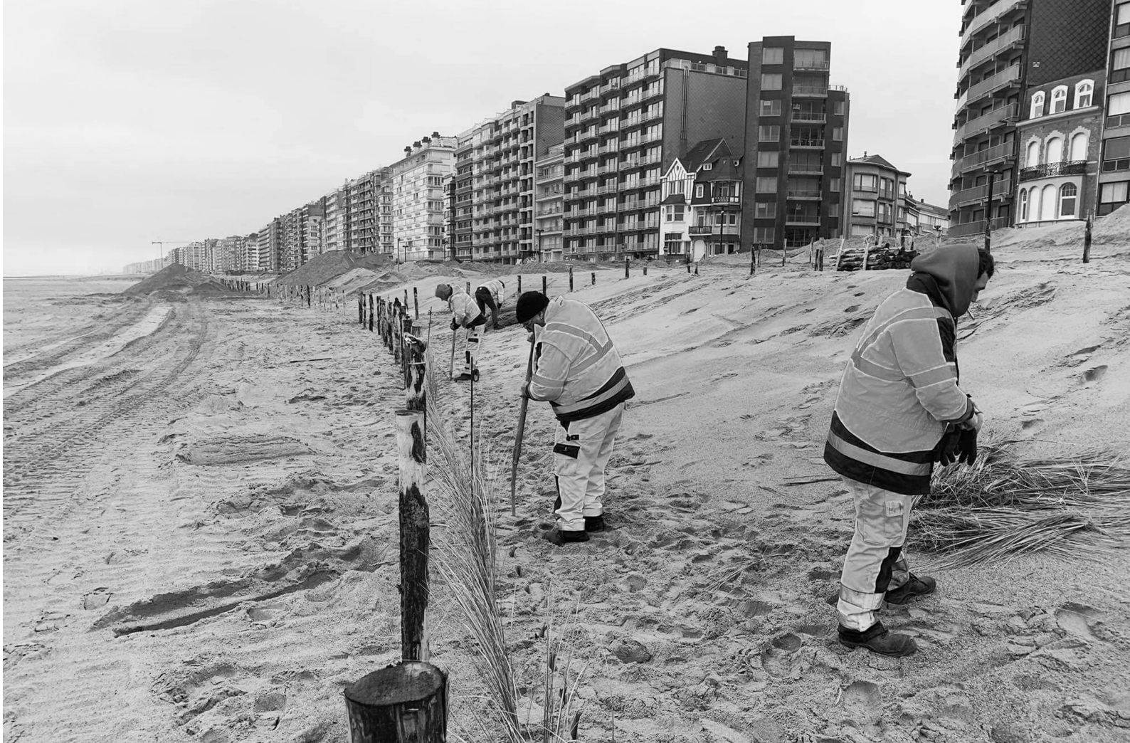
Planting of Marram grass and construction phases at the Middelkerke project site. Source: SARCC Project, 2022
